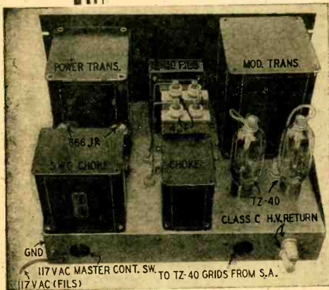
The power supply and modulator are mounted in one chassis unit.
